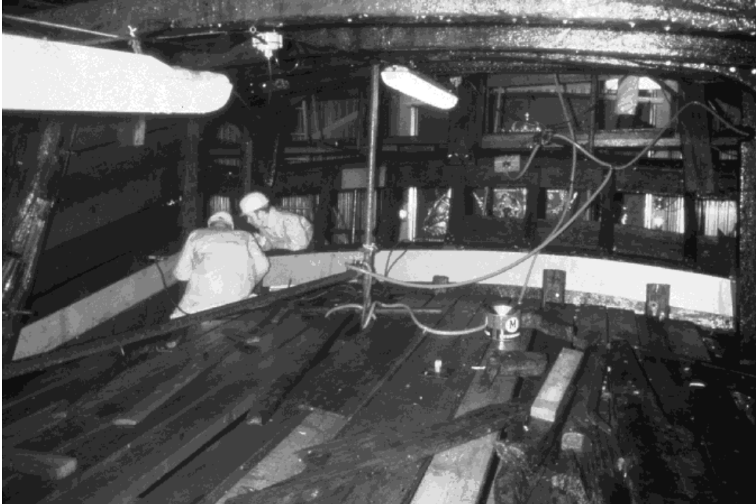
Figure 3-17 One of the steel constructions for support of the stern put into place (photo: Björn Hedin)
