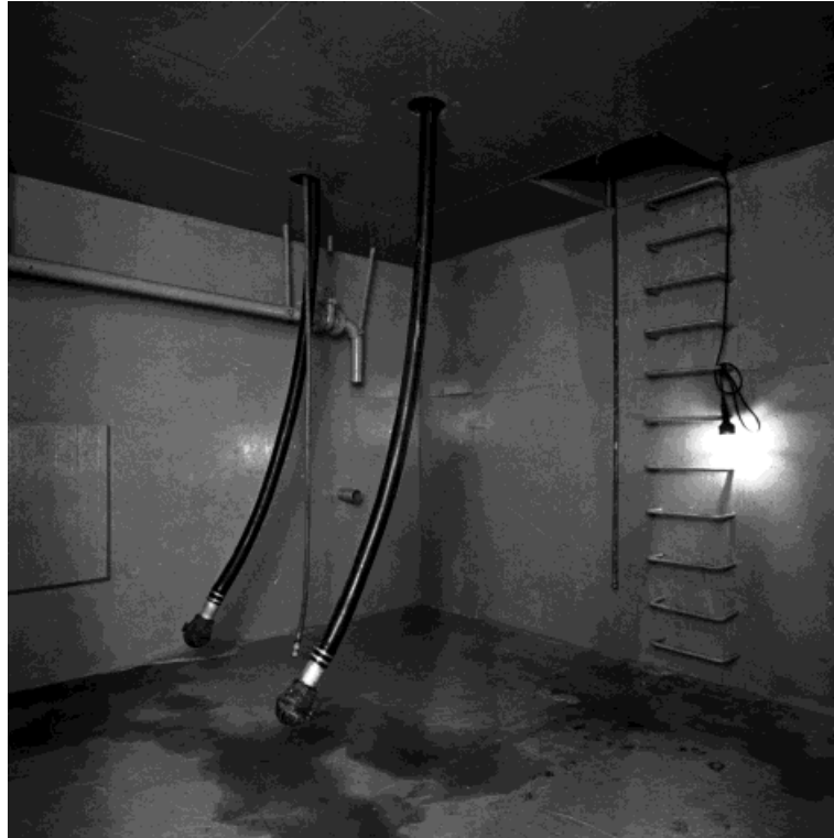
Figure 4-10 The preservation tank with rubber hose pipes for pumping the solution and pressure tubing for stirring. A sewer pipeline on the wall of the tank is for returning liquid (photo: Göran Sallstedt)
