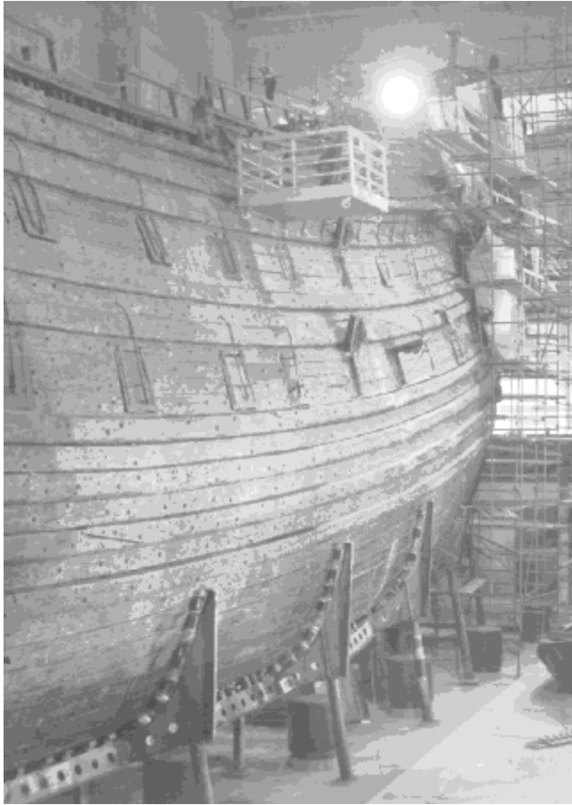
Figure 4-25 Work on the surface of the hull from a hanging work platform and scaffolding (photo: Sven Bengtsson)
