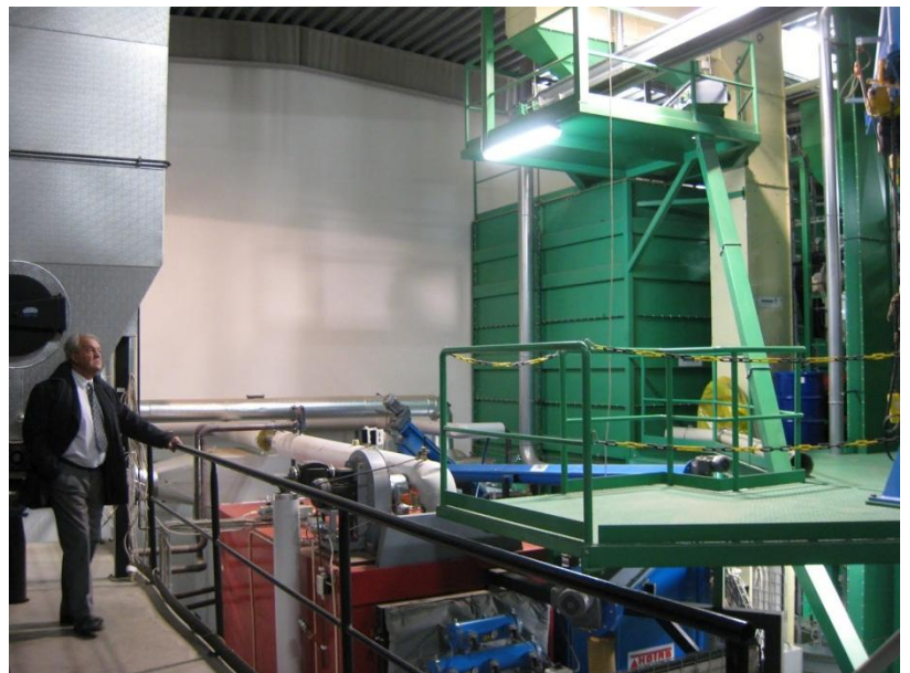
Figure 9: View over system solution at BIOAGRO
