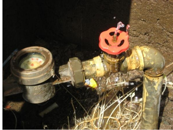
Figure 8.1 Well nr 4 leaking
