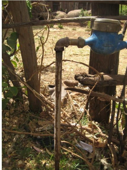
Figure 8.4 Leaking yard tap in Chitu
