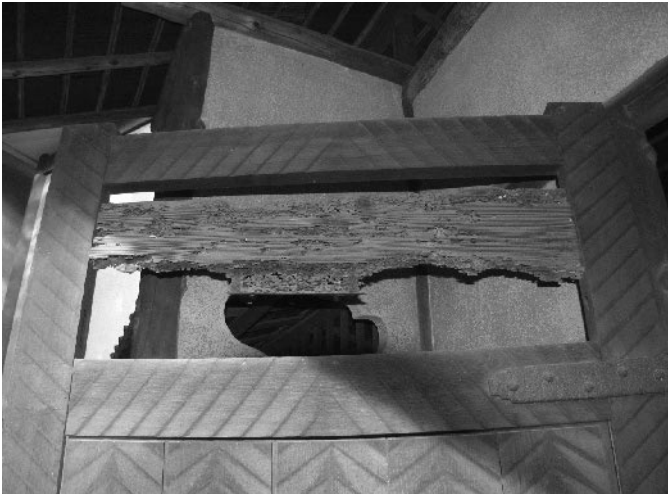
Figure 2.10: Decorative panel on Japanese gate cut from termite damaged wood. Gotō Museum garden, Tokyo.
