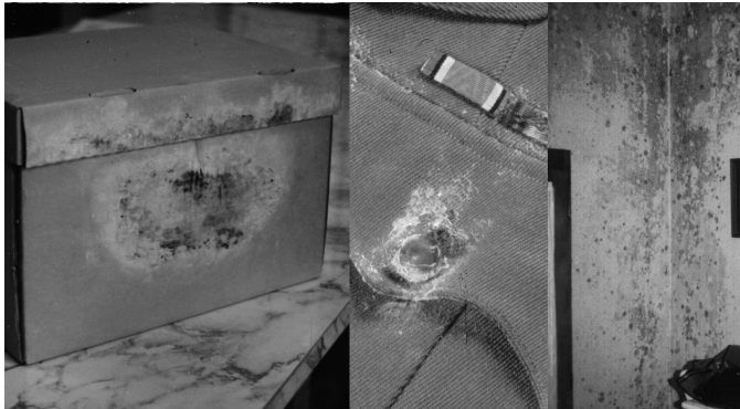
Figure 4.12: Three patterns of mould development: Left, bulging box against cold damp wall created convection tapering to diffusion controlled air gap resulting in moisture trap in central area. This also dries slower allowing more time for mould growth. Middle, leather button dressing increased mould nutrition on wool uniform allowing growth in shorter time than on surrounding wool. Right, winter heating of earth-floor basement generated moisture, stack effect drew it into upper stories, spring mould bloom concentrating in high cold corners with greatest adsorbed moisture (moist air rises). Photos left, centre CCI, right T. Stone.
