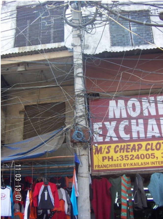
Figure 4.8: Tangled cables and wires in Central New Delhi.
