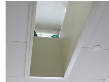
Openings between the floors makes it possible to wave to somebody upstairs.
