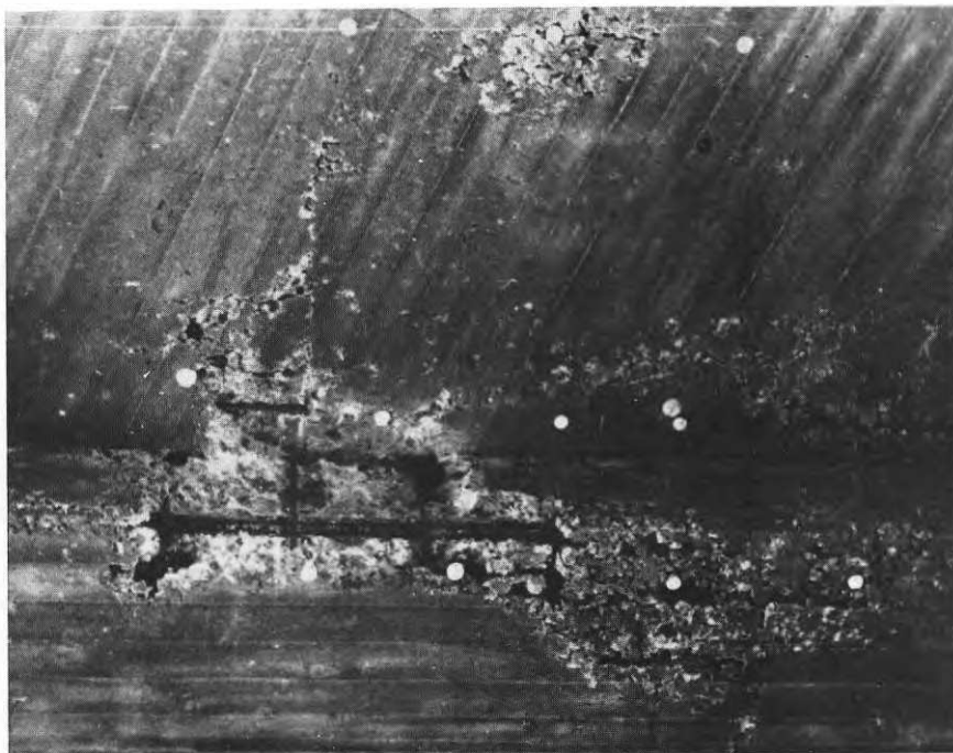
Example of honeycombing found on the soffit of a bridge after the formwork has been removed. This was repaired using the method described in the report.
