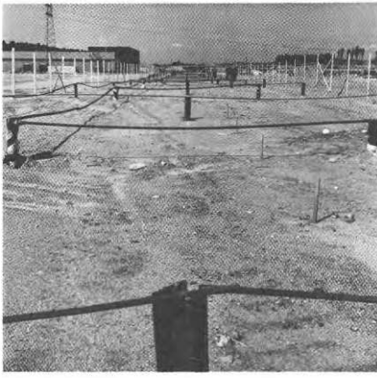
FIG. 1. Electro-osmotic stabilization of clay layer covered by 6—7 m thick sand fill at Scania Vabis, Södertälje. The electrodes of iron rails are mutually connected by reinforcing bars. The anodes and the reinforcing bars which connect the anodes are insulated with a plastic cover.
