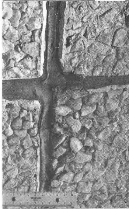
Fig. 84. Extrusion damage in oil-based jointing compound at a height of about 1 metre above ground.
