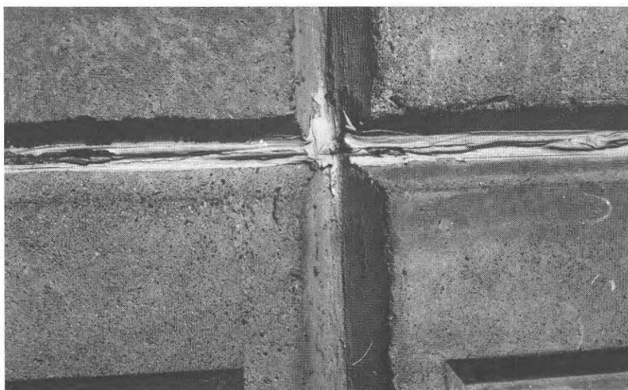
Fig. 78. A joint containing an oil-based compound after 11 years movement in the longitudinal direction of the joint (settlement). The jointing compound has dried considerably, a skin has formed and there are cracks at right angles to the folds.
