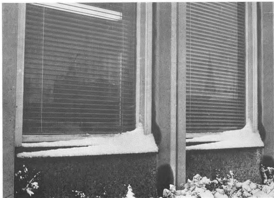
Fig. 53a. Window with deficient drainage. Water from the joint between the side pieces can run inwards at the corner of the frame. The drainage opening in the drainage channel of the bottom frame piece has been placed some distance from the corner, allowing formation of a pocket of water. The corresponding type of damage due to moisture is shown in Fig. 53b.
