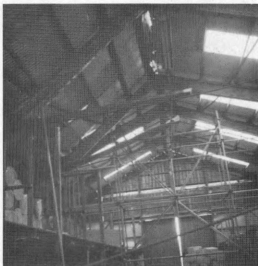
Fig.3 Brott i takbalkar
