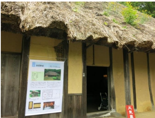
Fig 93. Roof on its process of decay.
