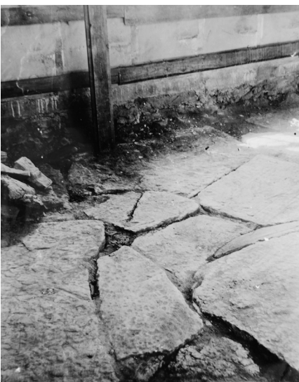
Fig. 2.3. Above , a view of the east gable in the nave in Forsby from the attic. The seam from a lower gable structure is visible. The mortar in the lower part contains small black particles of coal and is different from the mortar in the subsequent masonry on top. This may be connected to the remains of a limekiln filled with crushed limestone and charcoals, which was found outside the churchyard (Fornsök Forsby). The hole in the lower gable, which is likely from scaffolding, still contain small pieces of wood, and a sample has been identified as the species poplar wood (Seim et al 2015:42). Photo 2015. Left , a previous stone floor in the nave in Forsby, close to the north wall, which Norberg interpreted as original. Photo Norberg 1933, ATA.
