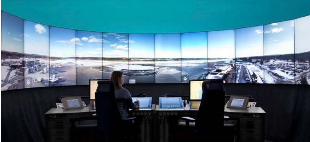
Figure 2. Remote tower system from SAAB Digital Air Traffic Solutions, Sweden (SAAB 2018).
