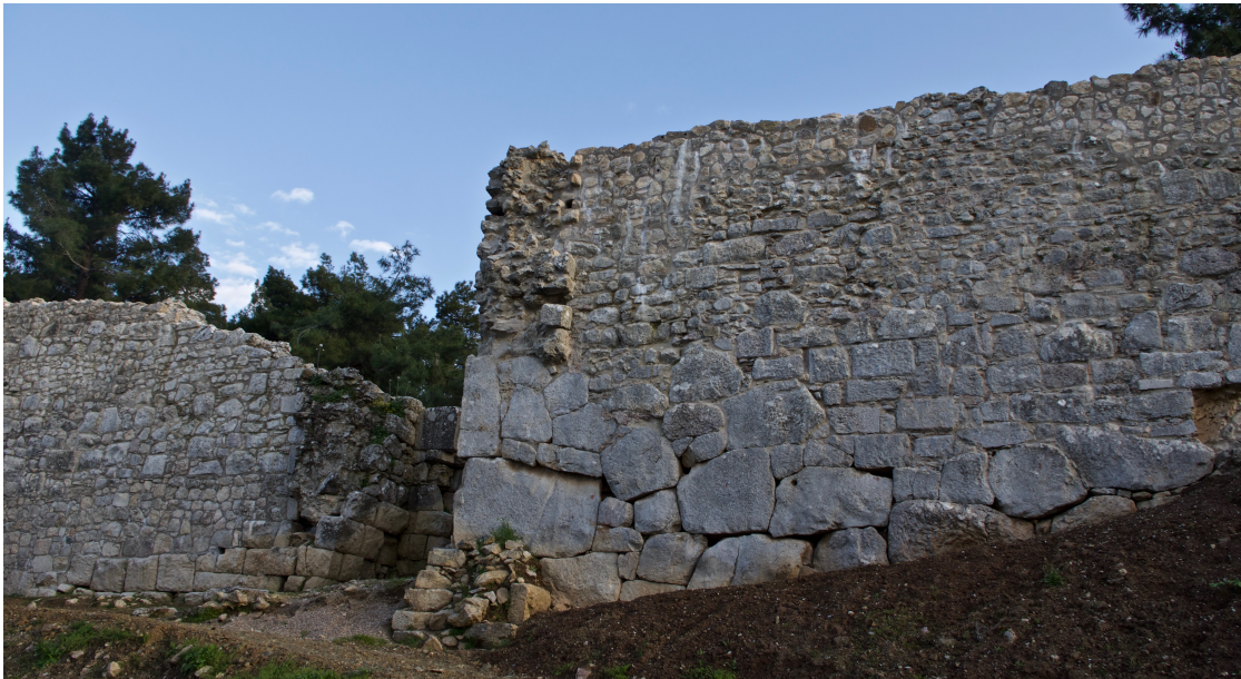
Figure 4.12: The recently restored cross-wall of the akropolis of Pharsalos ( B.1.14 ). The wall displays masonry of the pre-Poliorcetic, the Poliorcetic and the Late Roman-Byzantine phases. Photograph by Robin Rönnlund.
