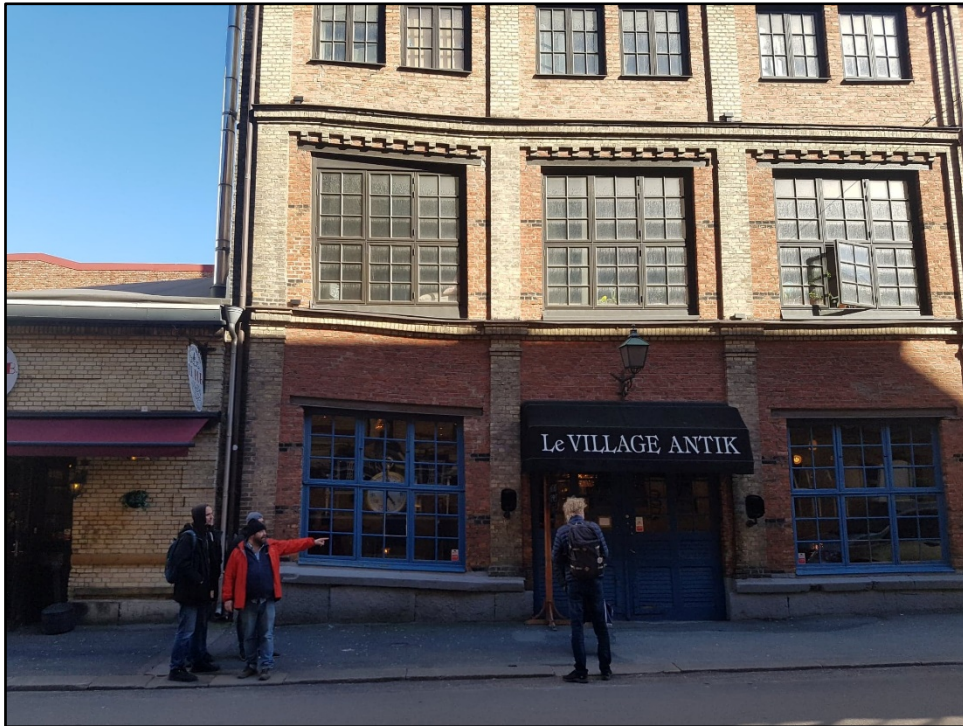
Figure 4. 1. A photo of Le Village shows severe settling in the left corner. However, on the second storey the settling is not as strong as in the ground level. Nordhemsgatan 24, Masthugget. Code: MH0811a
