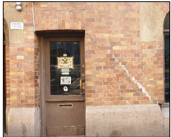
Figure 3. 2. This figure demonstrates a building with bricks sliding apart in the typical 45-degree pattern. Sveagatan 22. Code: KA0512
