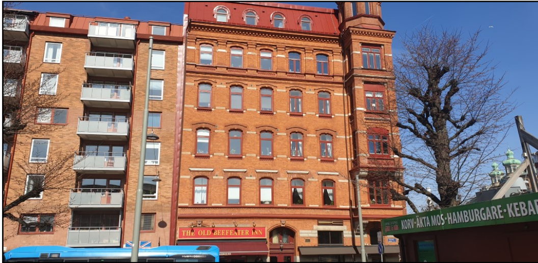
Figure 4.5. Seen from this angle the widened fire wall is evidence for the building leaning. Linnégatan 11 in Olivedal. Code: MH0204
