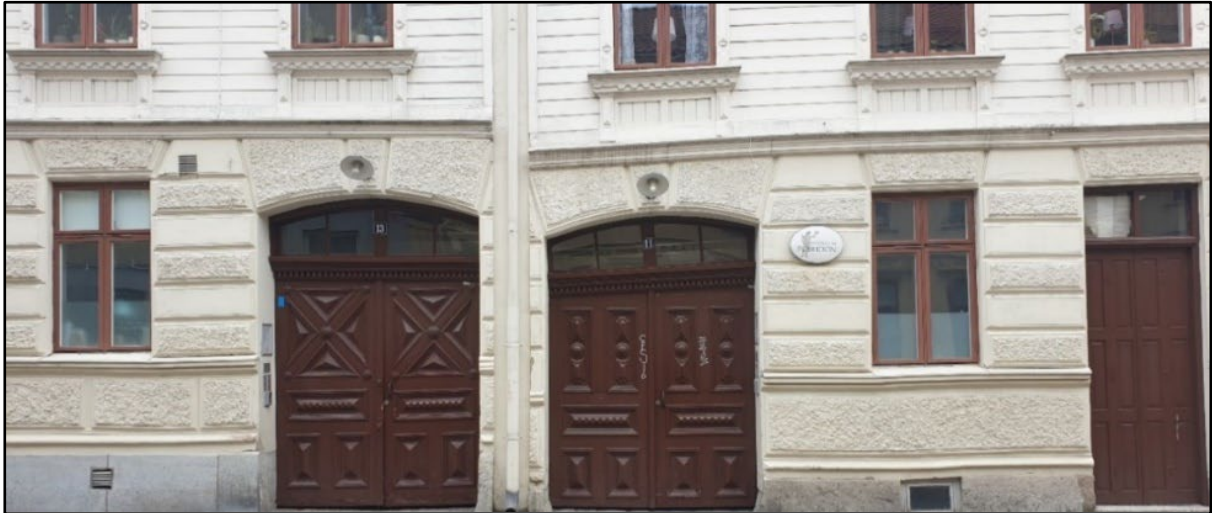
Figure 3. 5. Photo taken of deformed house skirting. The picture also shows an example of protracted vault. Västra Skansgatan 11, Haga. Code: HA1206e
