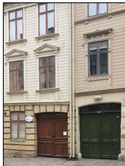
Figure 3. 10. Evidence of a sunken fire wall by looking on how the skirting deforms. Mellangatan 9, Haga. Code: HA1211c
