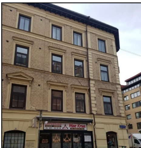
Figure 4.6. Sliding bricks can be seen from centre to right side but not on the left side. Andra långgatan 24, Code: MH0701b
