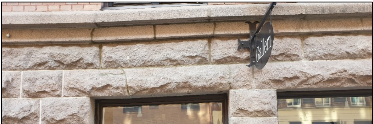
Figure 3. 6. This figure shows example of crushed house skirting. Plantagegatan 9, Masthugget. Code: MH0116
