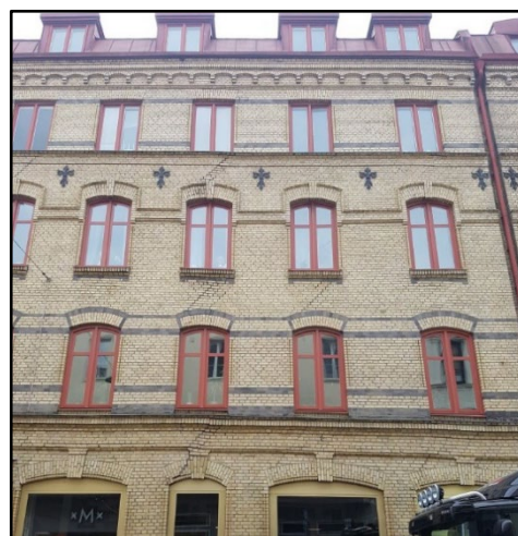
Figure 4. 7. Sliding bricks can be seen without any clear pattern. Andra Långgatan 4a, Code: MH0807
