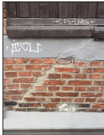
Figure 3. 8. On the top right a cracked and deformed windowsill is shown. Also, a pattern is seen along with the sliding bricks. Tredje Långgatan 13, Masthugget. Code: MH0811c
