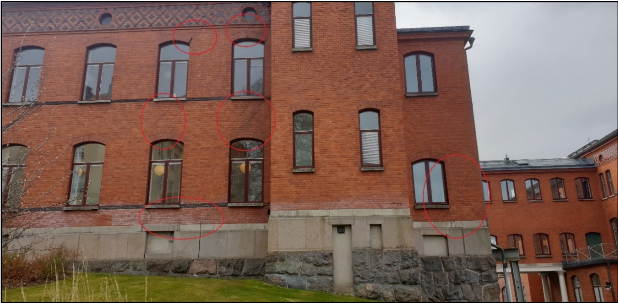
Figure 3. 13. This picture was taken from the north-east side, looking south-west and is marked with a yellow dot in fig 3.12. The building varies with depth from zero meters in the south-east part (left outside the picture) to depth of 5 meters in the north-west. The red rings enclose bricks sliding apart. Konstpedimins Väg 2, Code: KV2002c
