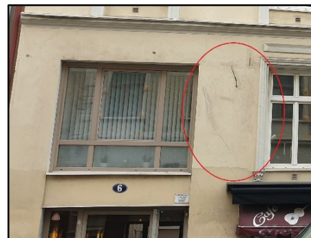
Figure 3. 4. Examples of cracks in a plastered facade at Andra Långgatan 6, Masthugget. Code: MH0804
