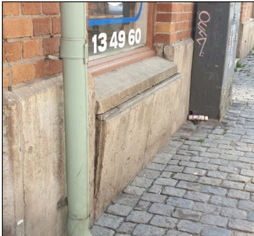
Figure 3. 11. Deformation of base stone found in Kommedantsängen. Majorsgatan 6. Code: KA0501
