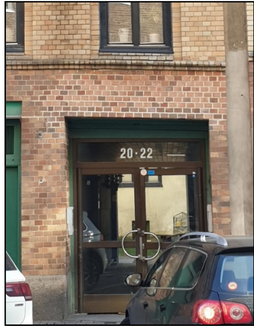
Figure 3. 9. Example of a protracted vault in a damaged area around kommedantsägen. Sveagatan 20-22. Code: KA0513
