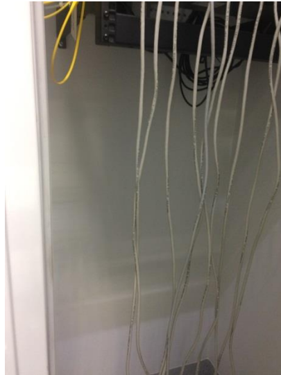
Figure 10. Inside the electrical cabinet, as a suggested location for a hatch.
