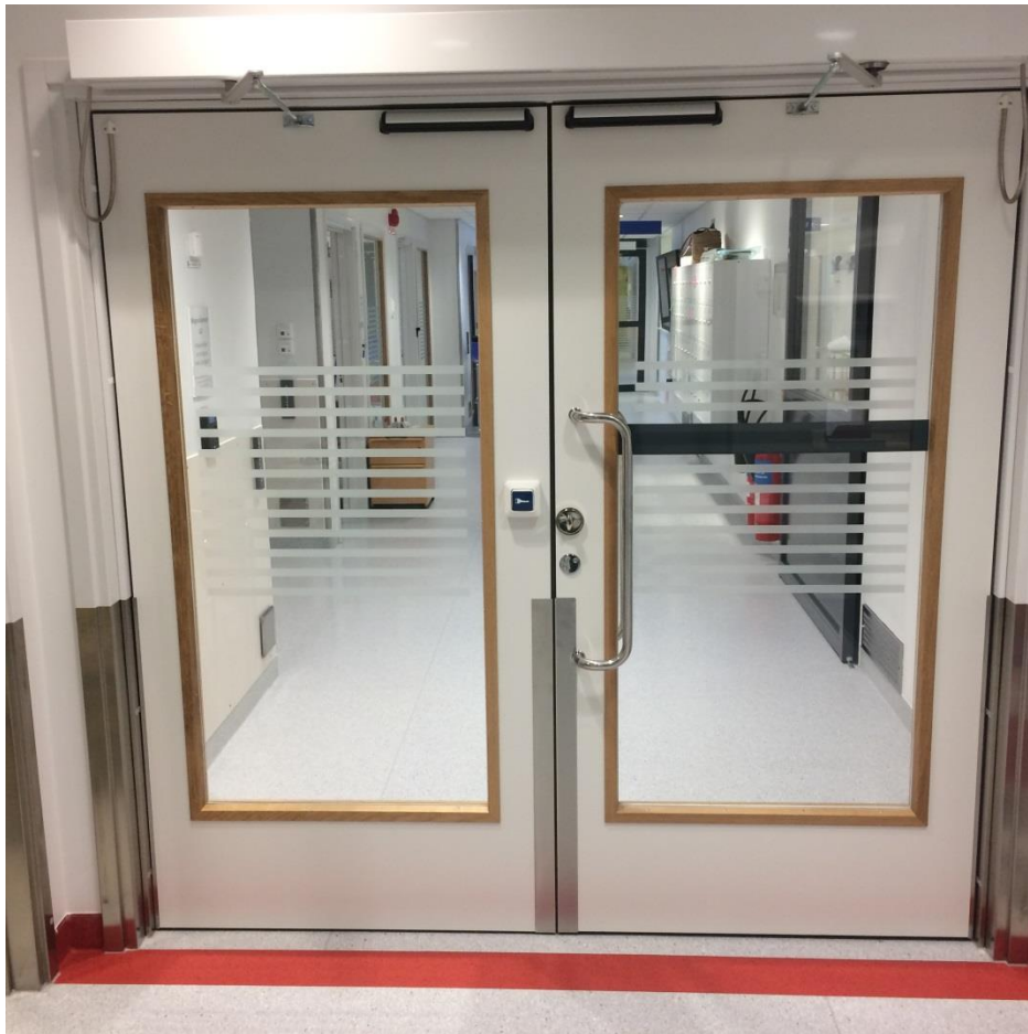
Figure 19. Final set of glass doors leading into the iMRI Hybrid OR area (viewed from inside).
