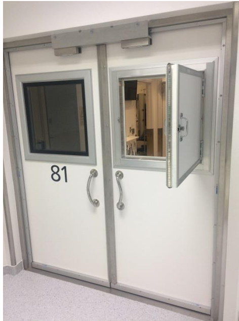
Figure 15. Hatch into the operating room in the open position.
