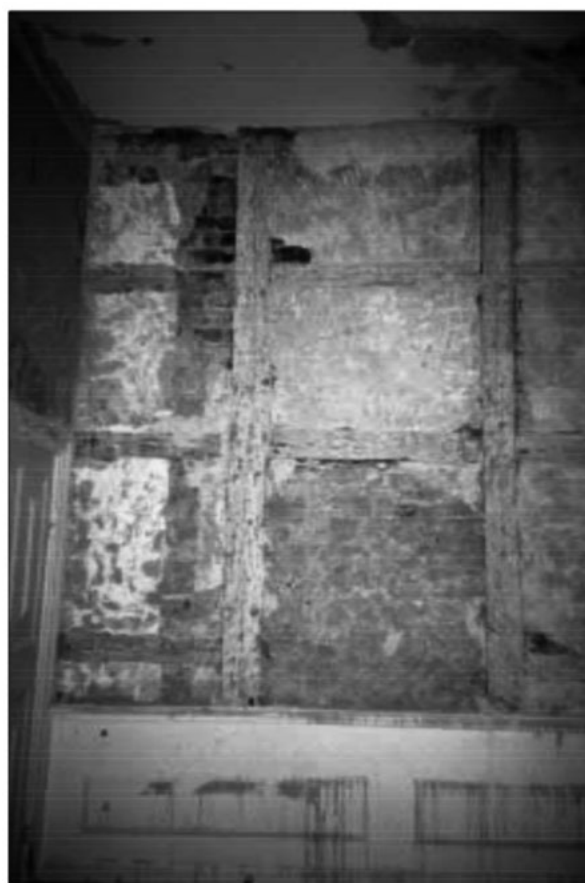
Figure 9 A timber-framed partition wall in Linköping Castle, with traces of a moved partition wall and a bricked-up door. (Modén 2003:36) Photo Eva Modén.
