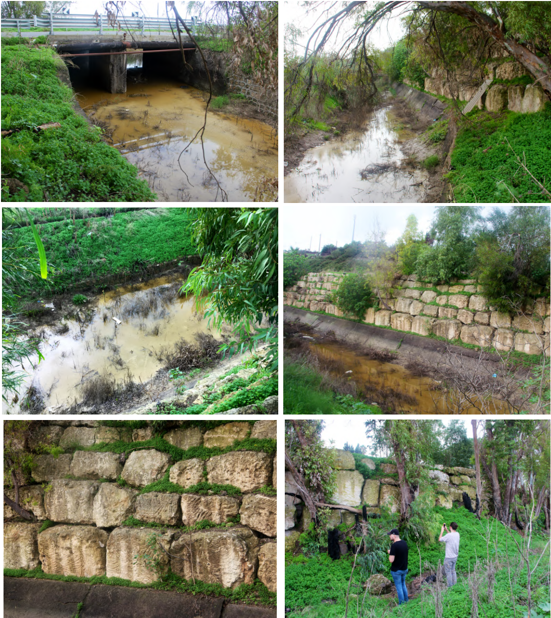
Fig. 19. (1) Canal, view of bridge-crossing on Stradale Coda Volpe. (2) Canal, view facing south to south-west. (3) Canal (direction north to south) turns east and bridges road going north to north-west after crossing (1.62m above sea level). (4) Walls facing east moving south. (5) Walls flanking canal, view facing west. (6) View of walls facing north-east and moving along road to south-east.
