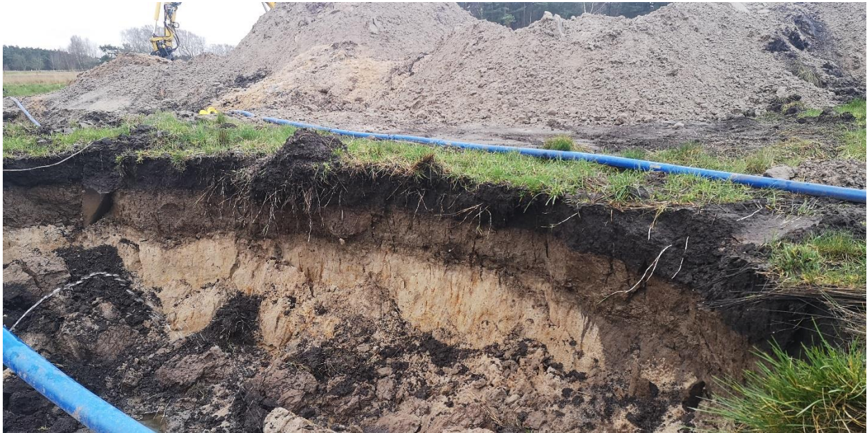
Figure 30. An excavation done west of the location for site H19001, the same stratigraphy was observed at the excavation as the one at site H19001. Rust precipitates can be seen in the sand.
