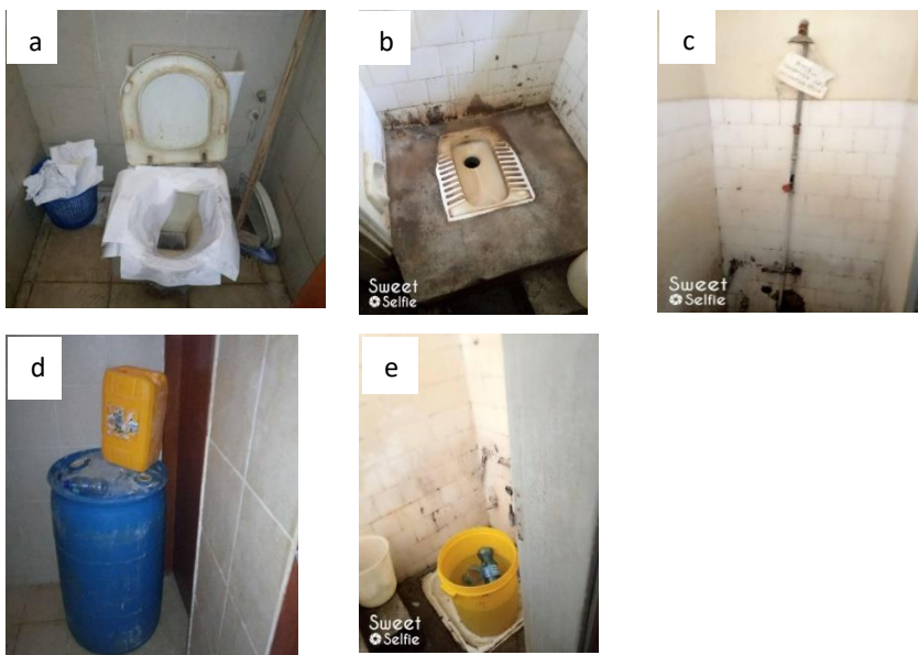
Picture 1:1 The toilet condition in one of health center located southern region Ethiopia with different types of toilet (Picture shared by the responder R4). a) flush toilet and b) squat toilet. Sometimes water is provided in a plastic barrel d) or container e).
